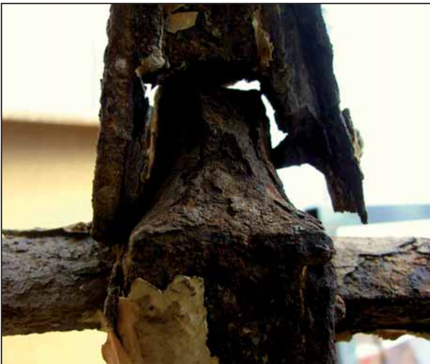
One of the extensively corroded joints of the housing
