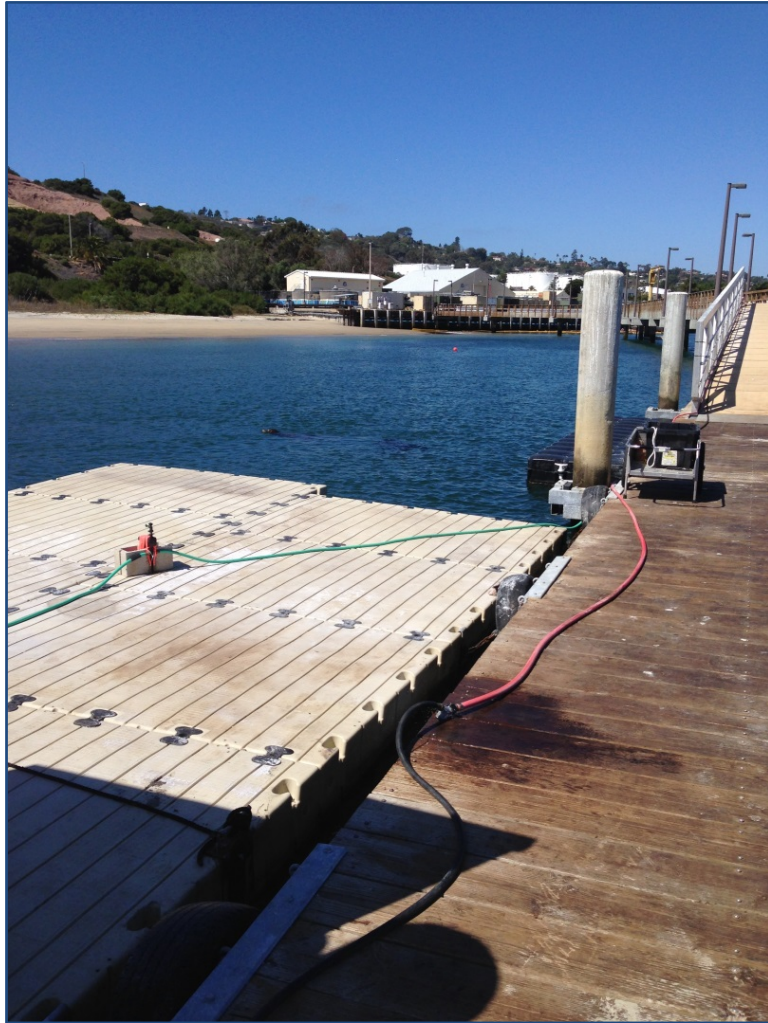
Photograph 20. Sprinkler with motion detector deployed on floating docks at Navy Base Point Loma, Point Loma, California.
