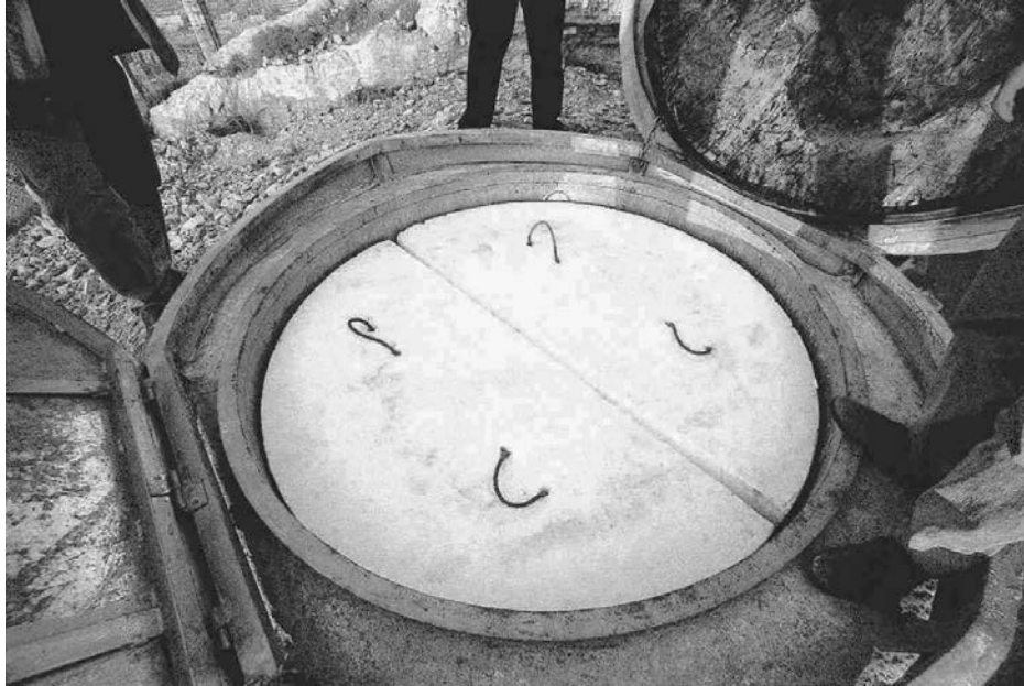
Fig. 7.41 Thermal cover of a seismic vault in two pieces made of thick styrofoam. The gaps between the cover and the vault walls and between both pieces must be tightly sealed.
