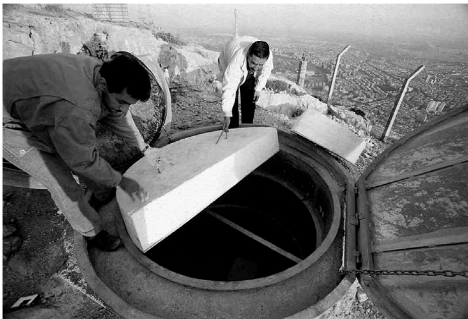
Fig. 7.42 Installing thermal cover in a seismic vault. In climates with large diurnal temperature changes the cover should be positioned lower in the vault where external ground temperature does not change significantly.
