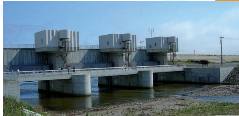
Water gate used to protect against tsunami waves on Okushiri Island, Japan. The gate begins to automatically close within seconds after earthquake shaking triggers its seismic sensors. Photo courtesy of ITIC.
