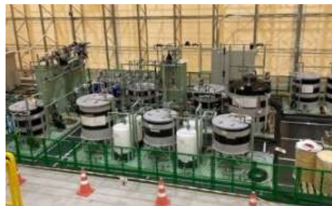
Adsorption process equipment (one of the three systems)
