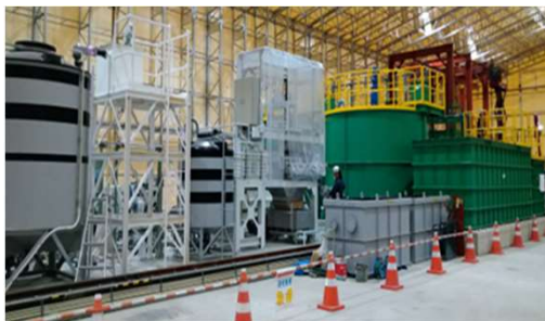
Cleaning process equipment
