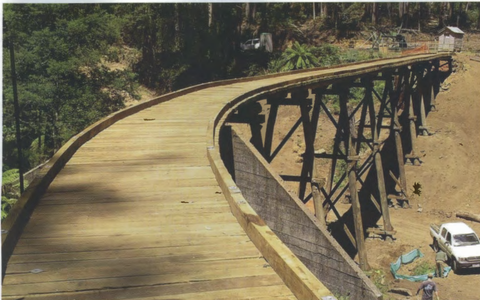
The completed 15,000 Syphon Bridge awaits the relaying of rails in February 2004. Photo: courtesy Bill Twitchett, DSE
