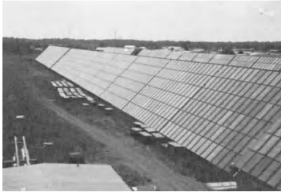
Figure 16.7.4 Collectors at the Green Bay water heating plant. Photo courtesy of R. Lane.
