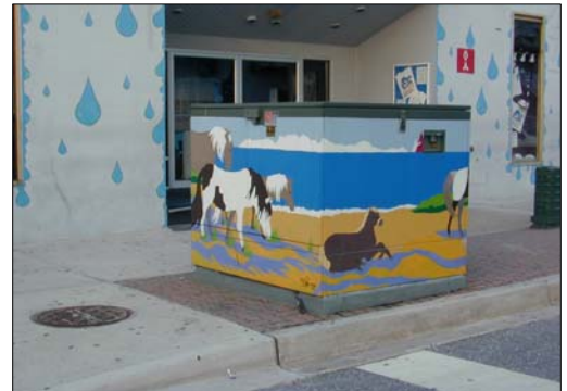
Transformer boxes decorated with artwork
