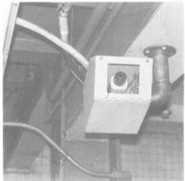
Figure 50. MTA-NYCT camera protective enclosure.
