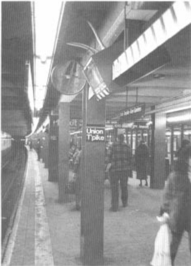
Figure 52. Union Turnpike station monitor installation.
