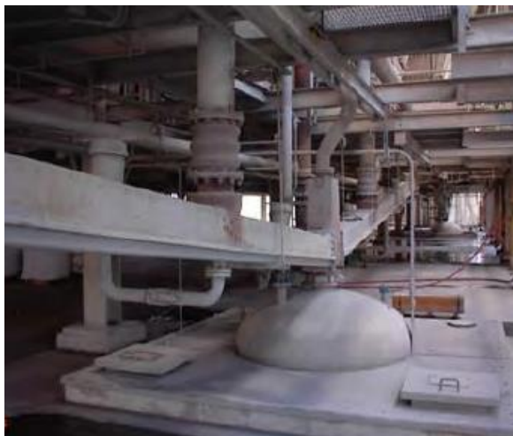
Air-assisted Gravity Conveyors below ESP
