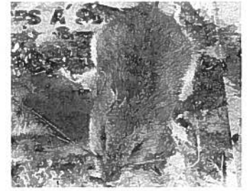
Mouse trapped while damaging attic insulation.
