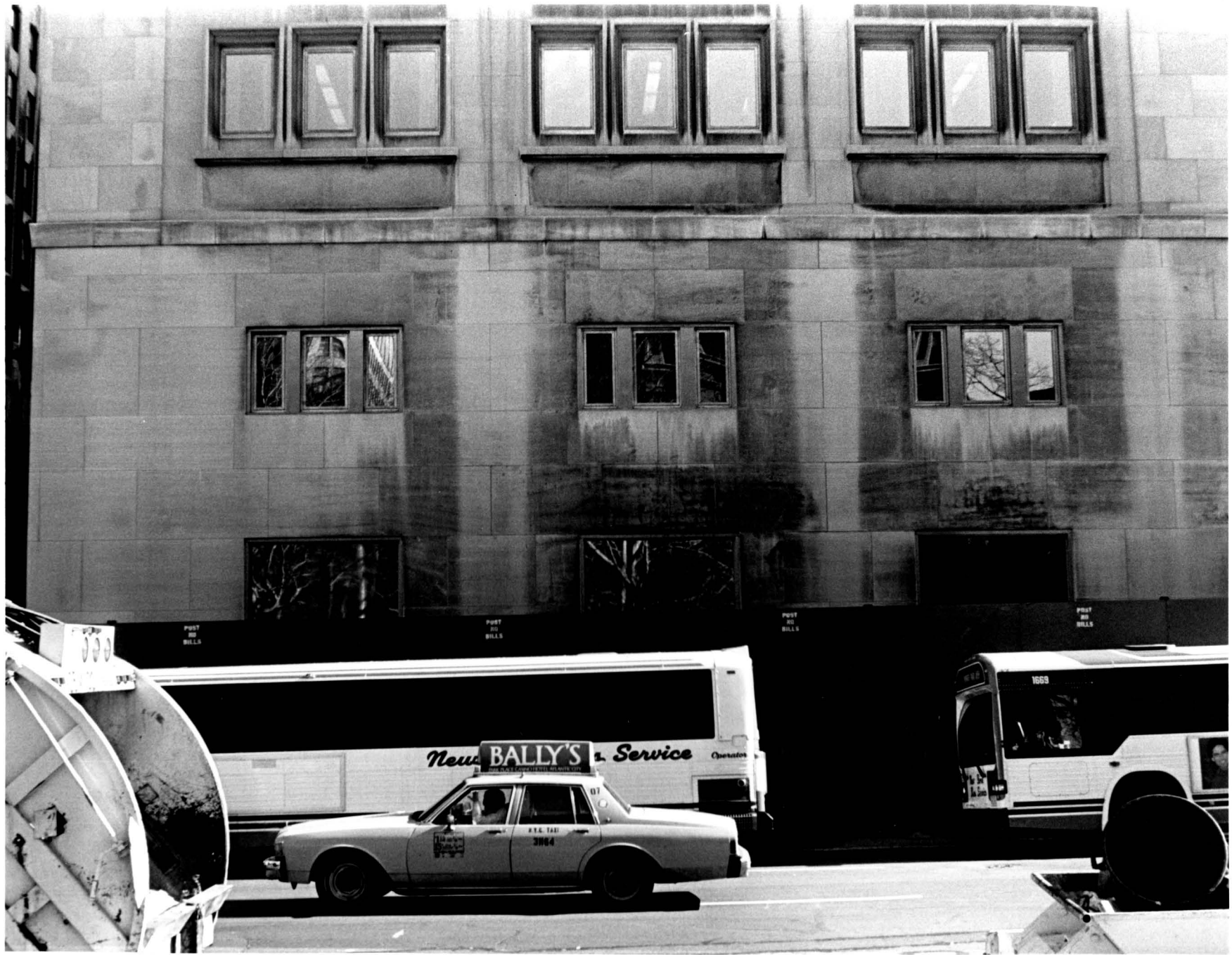
Plate 5. Base of the tower -- first, second and third stories, Madison Avenue elevation.
