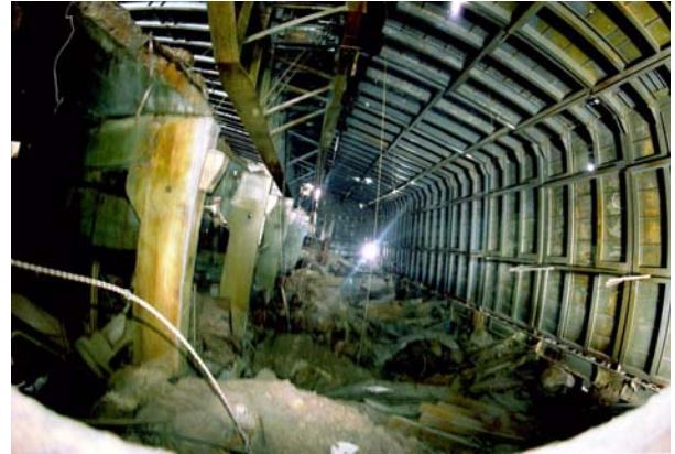
FIG. 7.3. Reactor room of unit 4 after the accident.
