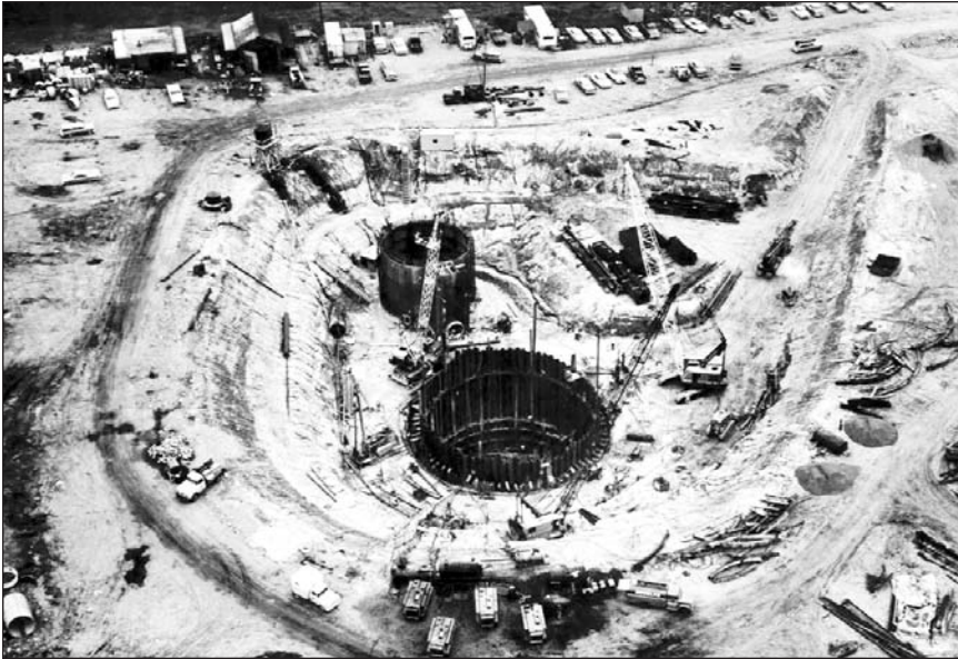
Construction site, early 1960s, for the Series F Atlas ICBM “silo-lift” launcher at Plattsburgh Air Force Base, New York. On a “silo-lift” launcher, the missile is stored vertically within a hardened, underground silo.
