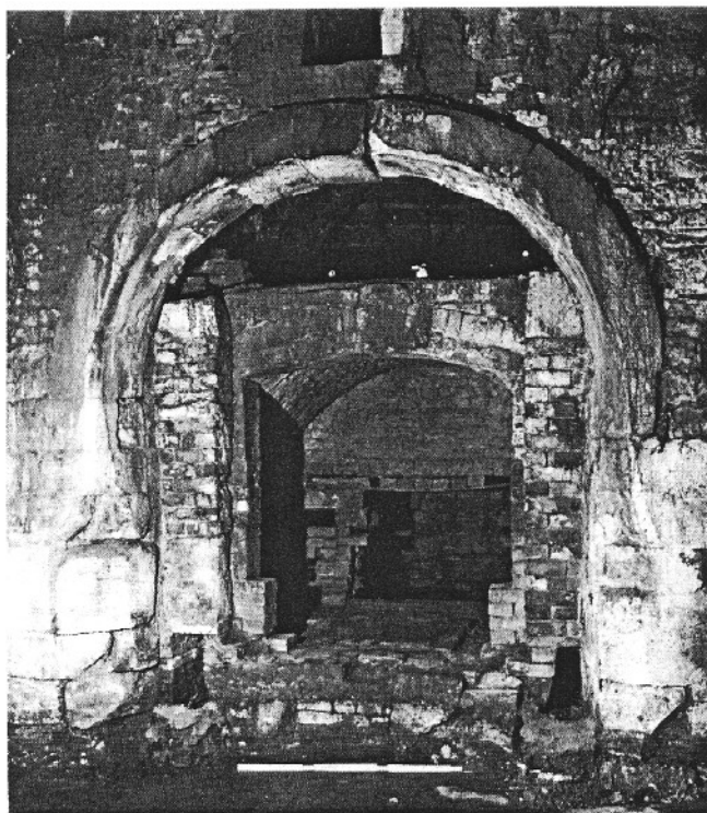
Fig. 10 Saltford annealing furnace from the front, before repair of the gaping hole in the rear face.
