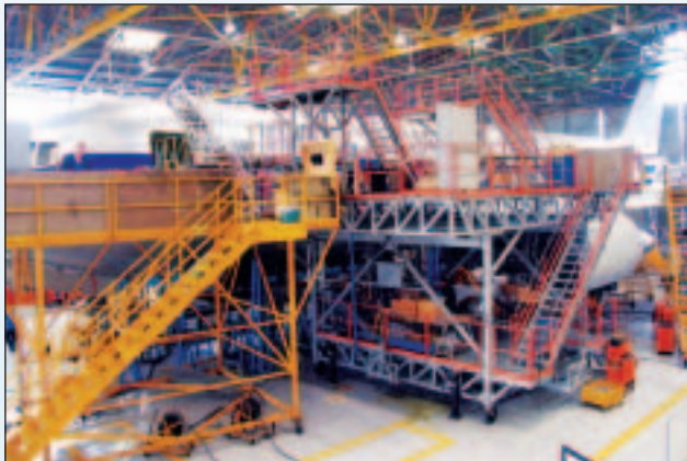
C-FGAJ in Tel Aviv Undergoing Conversion (Yes, There Is An Aircraft In There!)
