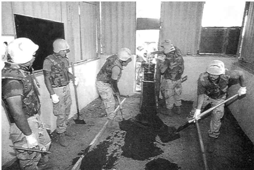
U.S. NAVY SEABEES FROM NAVAL MOBILE CONSTRUCTION BATTALION 1 POUR CONCRETE FLOORS IN CLASSROOMS AS PART OF A CIVIC ACTION PROGRAM OF OPERATION RESTORE HOPE.
