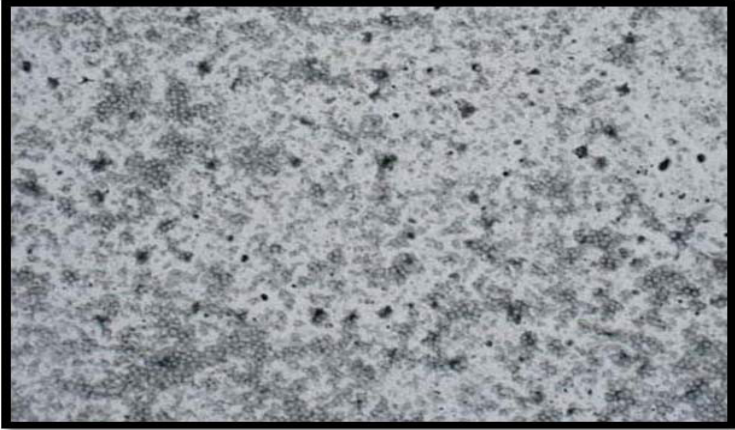
Figure E-6: Top View - Reflective Beads Applied that are Too Thin
