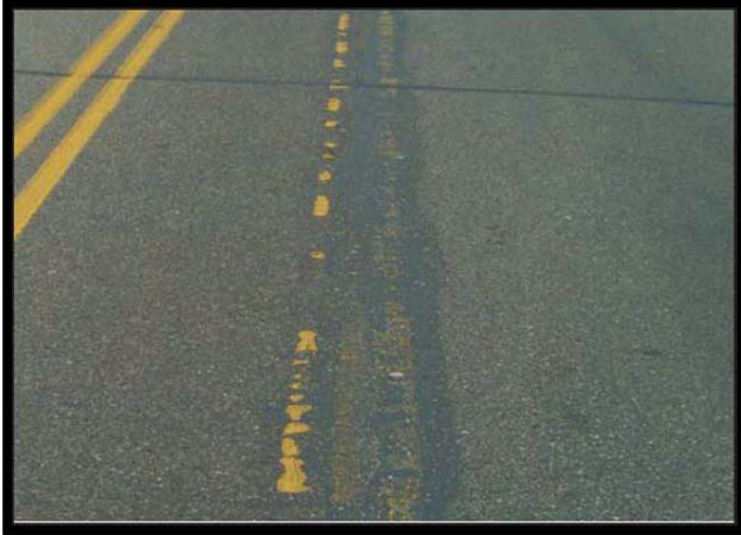
Figure N-3: Black Paint Wearing Off of Previous Marking
