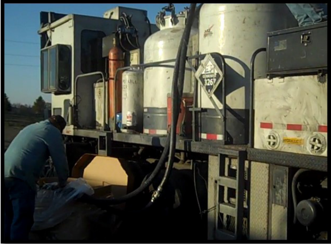
Figure P-11: Material Tanks (Refilling Beads)
