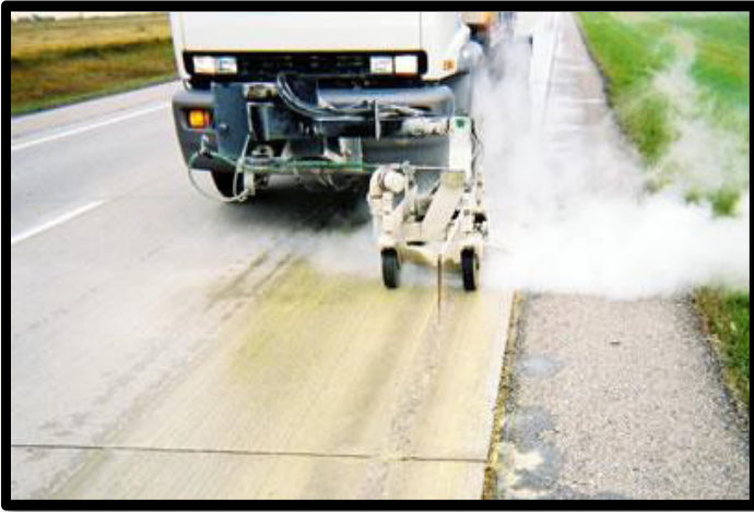
Figure J-1: Grooving operation prior to placement of the wet reflective material.
