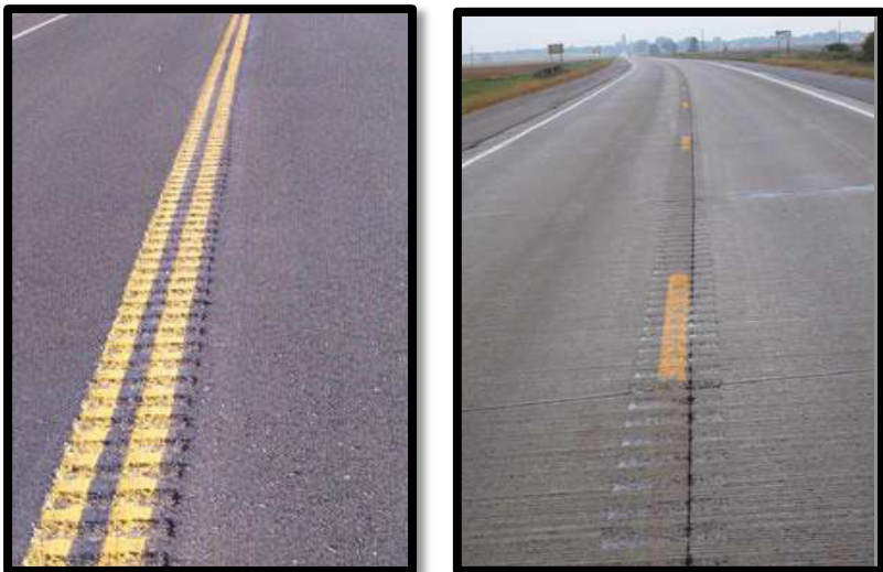
Figure K-2: Centerline Rumble Stripes
