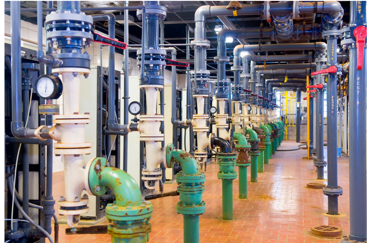
Interior of a drinking water treatment plant. Photo: EPA
