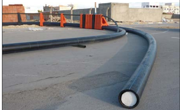
PLATE 43 Detail of the pipe end: the polystyrene cylinder is visible. Also the handrail is strung through the upper hole of the stanchions
