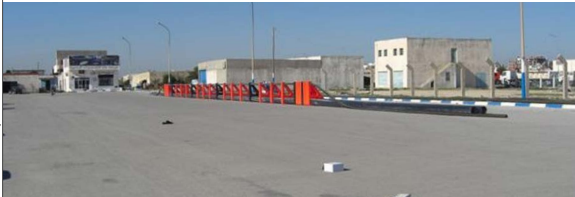
PLATE 41 The two main pipes after their construction. The pipes have already been inserted through the brackets, which are distributed along half of the pipe length. The handrail has been inserted as well
