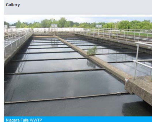
Niagara Falls Wastewater Treatment Plant High Rate Treatment, Canada
