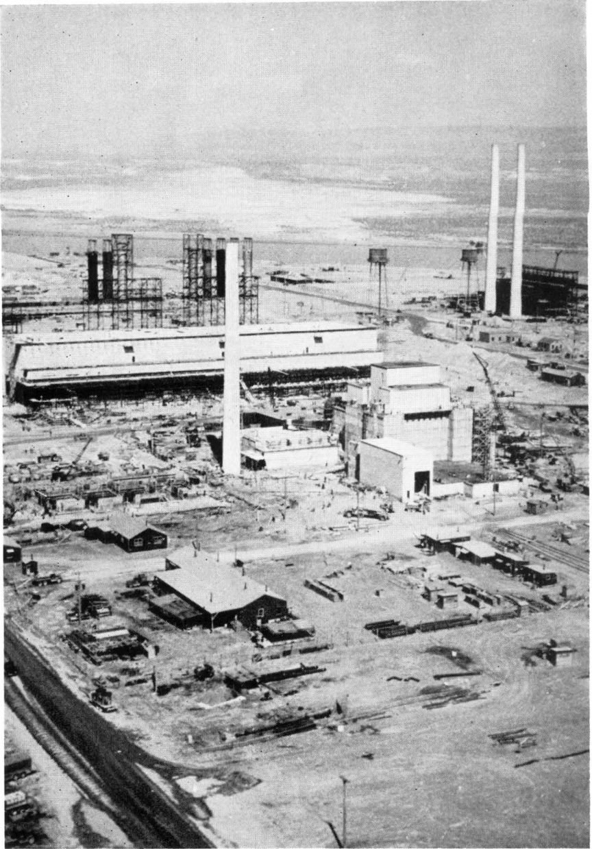
HANFORD D PILE AND SUPPORTING FACILITIES, JUNE 20, 1944 / The pile building, which towered 120 feet above the desert, is the concrete structure in the center. Behind it lies the water-treatment facilities. The Columbia River and the Wahluke Slope are in the background.
