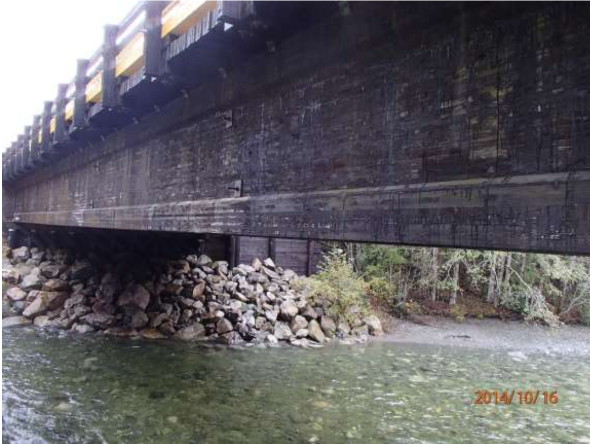
Figure 4-10: Heber River Bridge is a single-span, 34.5m (113ft) long consisting of four glulam I-beams and a transverse nail-laminated deck.
