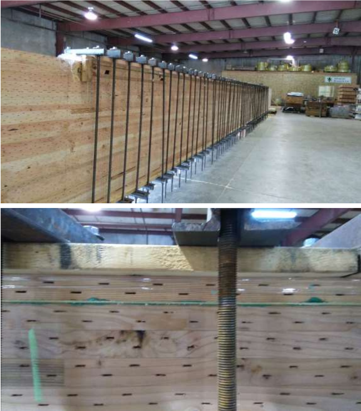
Figure 4-16: The glulam girders are reinforced with high-strength fiber on the tension face. This fiber-reinforcing is installed in the shop prior to assembling the structure.
