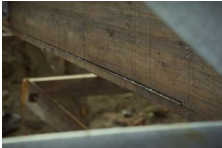
Figure 4-28: The glulam girders are reinforced with a layer of fiber-reinforced polymer (FiRP®) which permitted a significant reduction in the volume of wood required compared to an unreinforced bridge. This bridge has been in service since the early 1990's.
