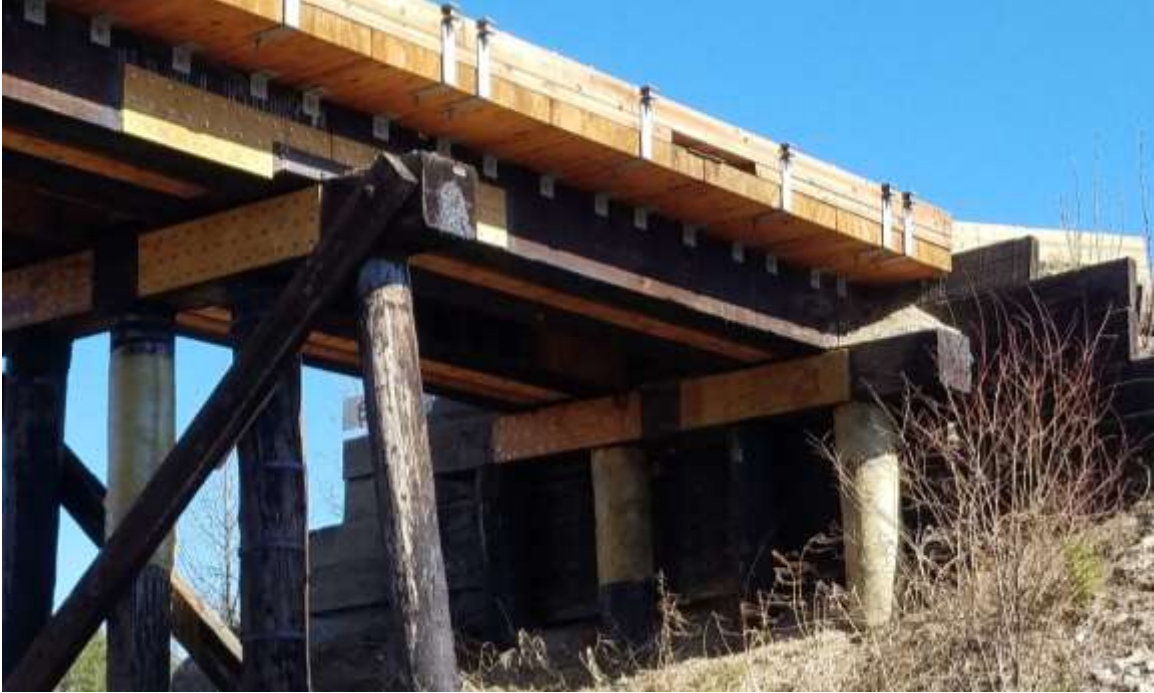
Figure 4-19: The Existing piles, caps, and chords were reinforced with high-strength fiber to restore capacity that had been lost due to decay. The old deck was removed and replaced with a new transverse glulam timber deck and curb.
