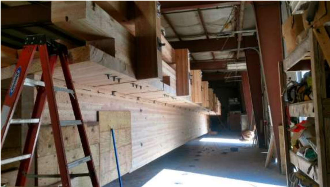
Figure 4-17: All timber components are fabricated and pre-assembled in the shop prior to preservative treatment. This dry-fit process helps avoid any field modifications that might compromise the preservative treatment layer. The bridge is then disassembled and the components are pressure-treated. They will later be shipped to the site for final assembly. The bridge incorporates an all timber TL4 truck crash proof rail system. The abutments are totally constructed of wood as well. The use of timber abutments versus concrete allows a much shorter construction period as there are no cure time issues relating to placement of the superstructure.
