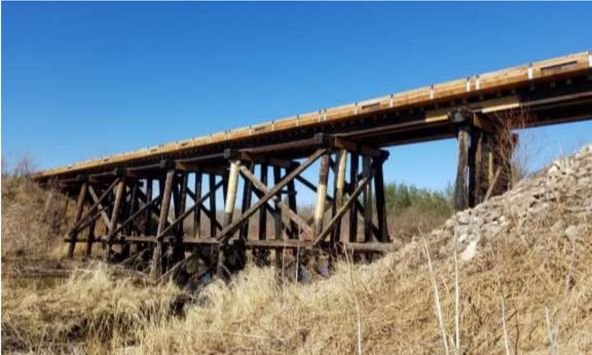
Figure 4-18: Meadow Lake Bridge is a conversion of a decommissioned railroad trestle to be used as a forestry bridge.
