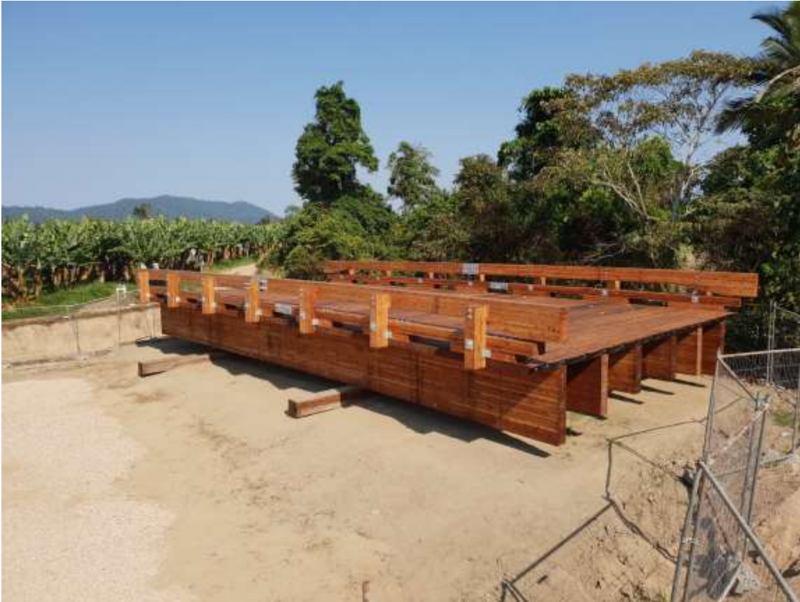
Figure 4-38: Cowley Creek Bridge, fully assembled and ready to be installed as soon as the foundation upgrades are completed.
