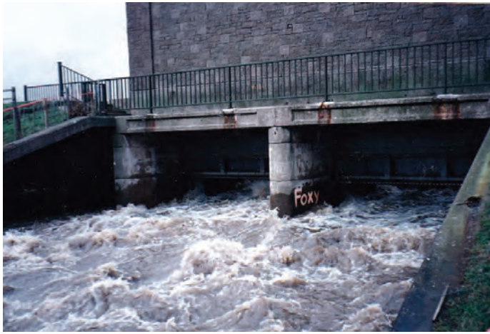
Figure 9: Floodwaters being released from the Mersey (behind the weir structure in this picture) into Sale Water Park through the basin inlet near the Jackson's Boat Public House.
