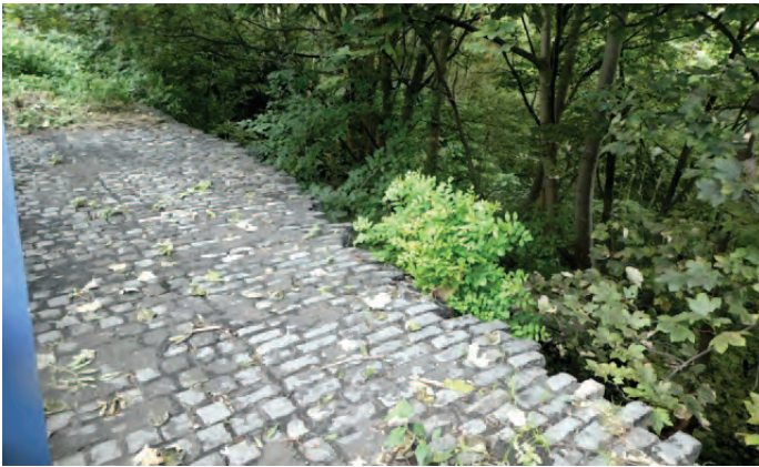
Figure 30: The collapsing continuation of Great Clowes Street.
