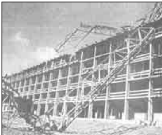
▲ Cara Inn Damaged
