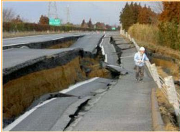
Just after earthquake occurred
