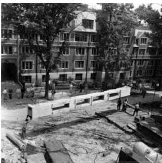
IMAGE SIXTEEN: Construction photo, Alfred Newton Richards Medical Research Laboratories, University of Pennsylvania, Philadelphia, Pennsylvania. The Architectural Archives, University of Pennsylvania. Photograph: Marshall D. Meyers
