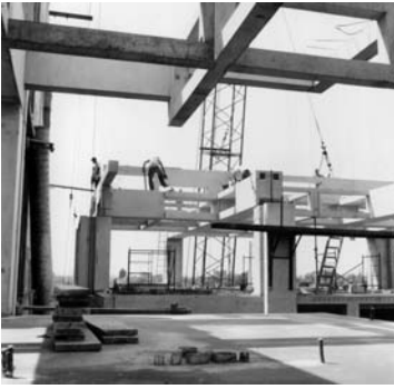
IMAGE EIGHTEEN: Construction photo, Alfred Newton Richards Medical Research Laboratories, University of Pennsylvania, Philadelphia, Pennsylvania. The Architectural Archives, University of Pennsylvania. Photograph: Marshall D. Meyers
