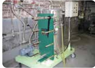
Heat exchanger (for pasteurization)
