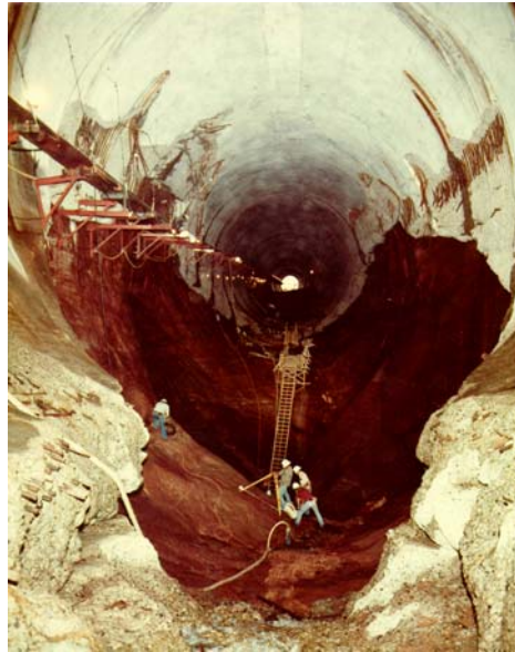
Figure 4. Damage to Glen Canyon Dam left spillway in 1983. The “big hole” was 11 meters deep.
