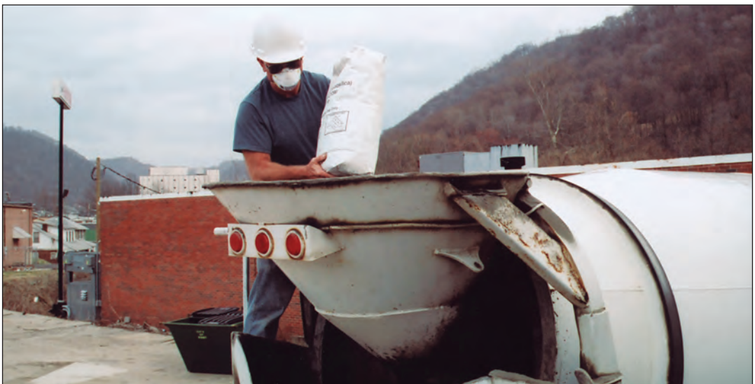
FIGURE 6.6. Adding repulpable bags of densified silica fume directly to truck mixer. See Section 6.3 for precautions regarding unopened bags. Note the use of a dust mask and safety glasses. See Chapter 9 for personal safety recommendations.
