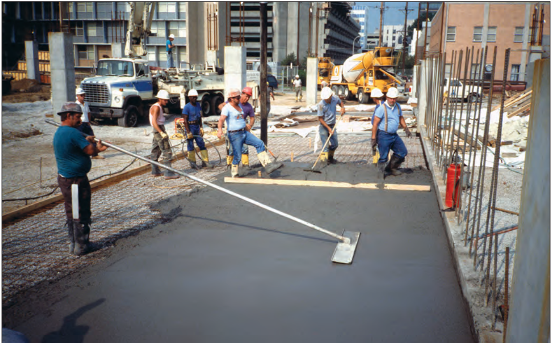
FIGURE 7.14. Conducting a trial placement using the one-step finishing process using a slab on ground in the actual structure. Note that placing the wire mesh on the bottom of the slab is not recommended practice.
