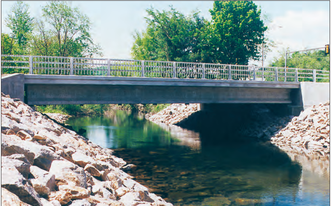
FIGURE 3.8. High-performance concrete bridge. In this bridge in New Hampshire, high-strength concrete was used to reduce the number of girders required for the structure. For more information on this bridge, see the article by Wasczik (1999).
