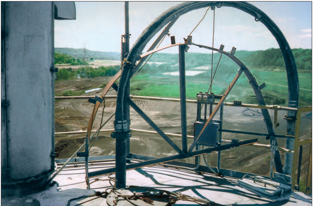
FIGURE 6.4C. Rubber fill hose connected to steel pipe on silo top. Note support frame for rubber hose being fabricated.
