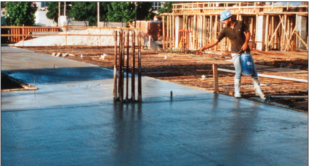
FIGURE 7.4. Applying evaporation retarder to silica-fume concrete to prevent loss of moisture before curing begins.
