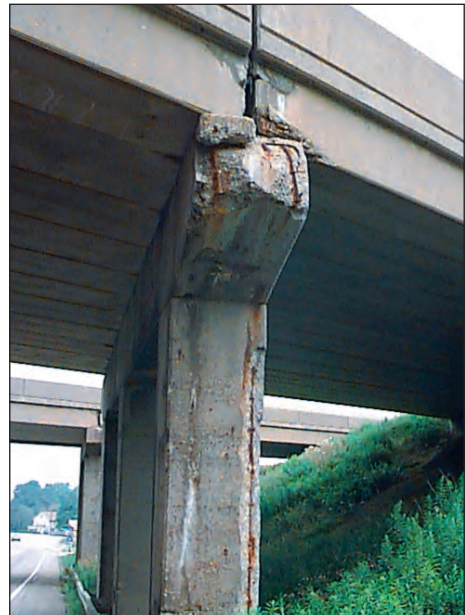
FIGURE 3.13. Corrosion damage to a highway overpass. Note that chlorides have apparently run off of the deck and onto this pier. Structural elements, as well as decks, should be protected.
