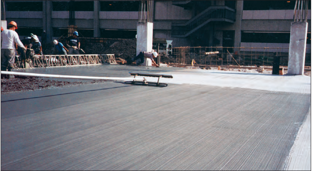
FIGURE 7.17B. This photo shows a finishing tool that is a combination of a float and a broom. In one direction, it serves as a float. In the other direction, it serves as a broom.
