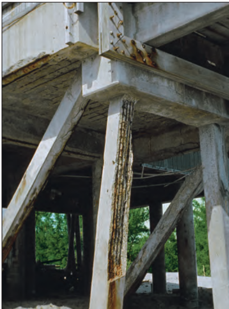
FIGURE 3.12. Corrosion damage to a marine structure.
