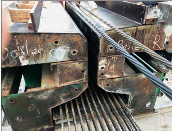
FIGURE 3.25A. Cross-section of a beam ready to receive UHPC. Note the minimized concrete volume and absence of secondary reinforcing steel.
