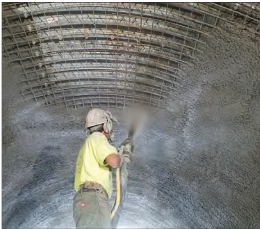
FIGURE 3.20A. Overhead application of silica-fume shotcrete. Because of its increased cohesion, silica-fume shotcrete has much less rebound and allows for greater lift thickness when shooting overhead than shotcrete without silica fume.
