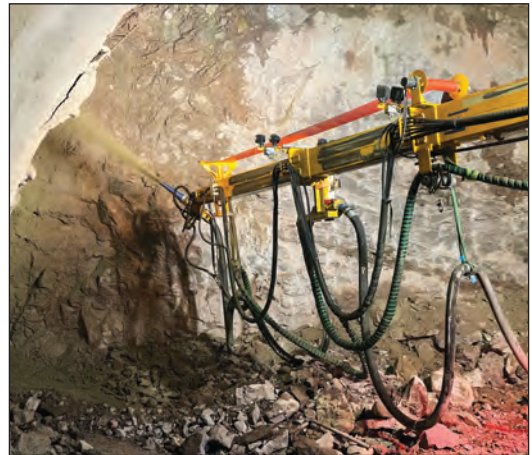
FIGURE 3.20B. Robotic application of silica-fume shotcrete for ground support. This process is used with and without steel fibers for additional flexural performance.
