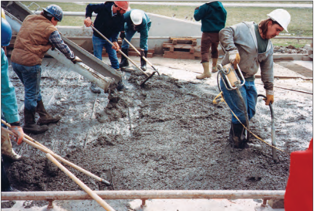
FIGURE 7.8. Silica-fume concrete being placed on the deck. Note the use of the vibrator to provide additional consolidation to that provided by the finishing machine.
