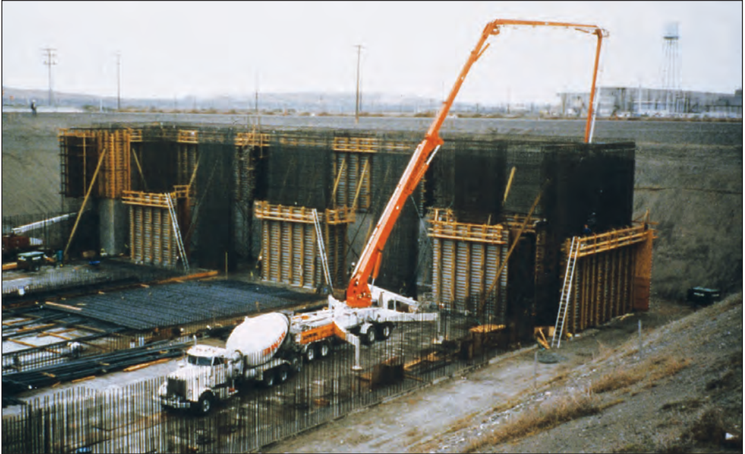
FIGURE 3.18. Concrete containing portland cement, fly ash, and silica fume being placed. The fly ash was used to control heat of hydration, while the silica fume provided early strength required for stripping forms. For more information on this project, see the article by Holland (1998).
