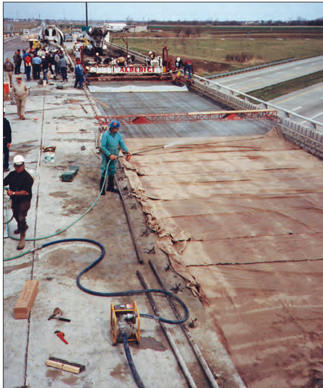
FIGURE 7.11A. Curing silica fume bridge deck. Curing is following placement and finishing without any delay.
