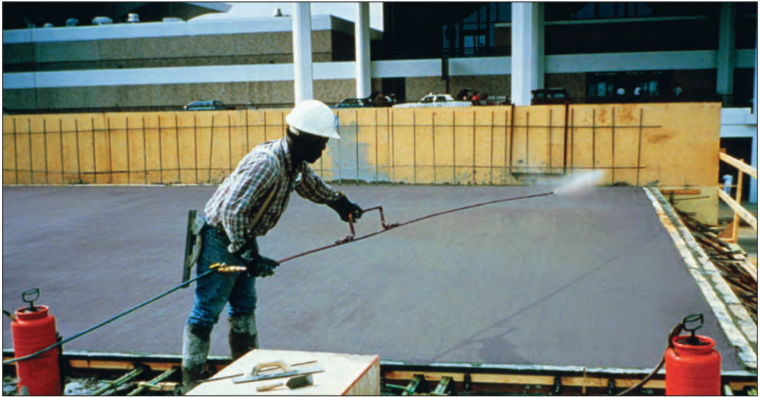
FIGURE 7.18. Curing compound is being applied to silica-fume concrete in a parking structure shortly after brooming. In many cases, the use of curing compound is the preliminary curing method; it is intended to protect the concrete until it gains enough strength to allow placing wet curing materials on the deck without marring the surface. On this particular project, wet burlap and plastic sheeting were used for the final curing.
