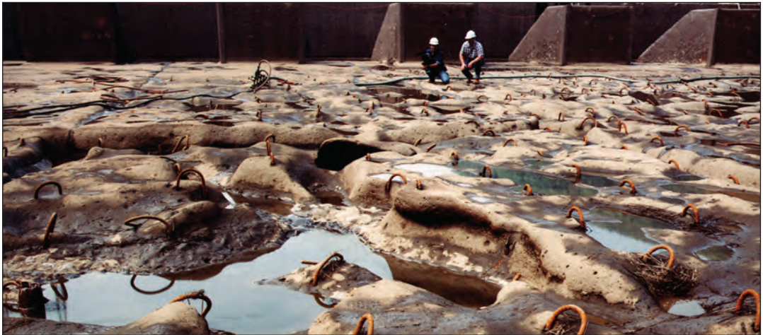
FIGURE 3.17. Abrasion-erosion damaged concrete. This structure was repaired using high-strength silica-fume concrete with a specified compressive strength of 86 MPa. For more information on this project, see the article by Holland et al. (1986).
