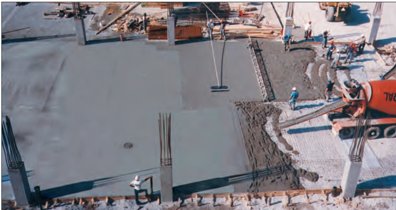
FIGURE 7.12. One-pass finishing. Concrete is being placed, screeded, floated, textured, and cured without any waiting between operations.
