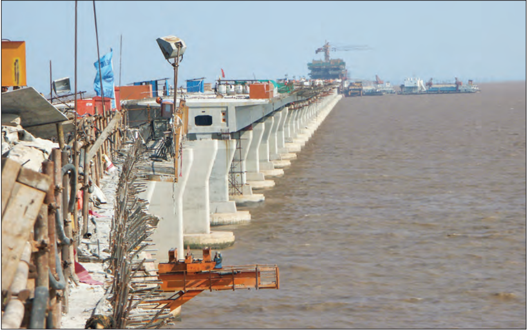
FIGURE 3.16. Specifications of the 32.5 km long East Sea Bridge between Shanghai Harbor and Little Yangshan Island required a 100-year service life. Quaternary high-performance concrete including portland cement, silica fume, fly ash and slag cement was utilized for the 35 MPa and 50 MPa structural designs, yielding a chloride diffusion coefficient reduction up to 75 percent over conventional concrete and very low rapid chloride permeability below 750 coulombs.
