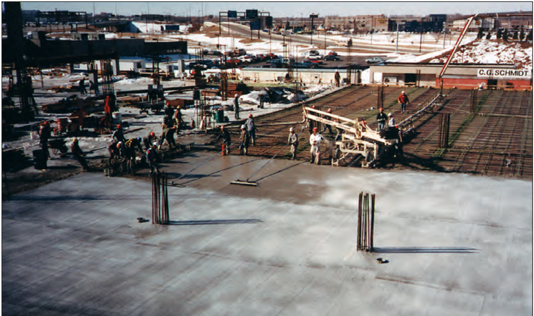
FIGURE 3.3. One-pass finishing of silica-fume concrete in a parking structure. Placing, finishing, texturing, and curing are done as a continuous process.
