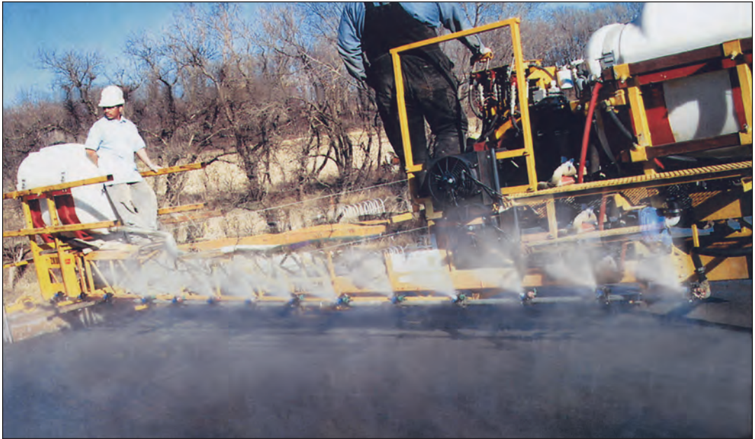
FIGURE 7.5B. Fogging equipment mounted on paving machine. The fog nozzles are pointed upward so moisture is not added to the concrete surface.
