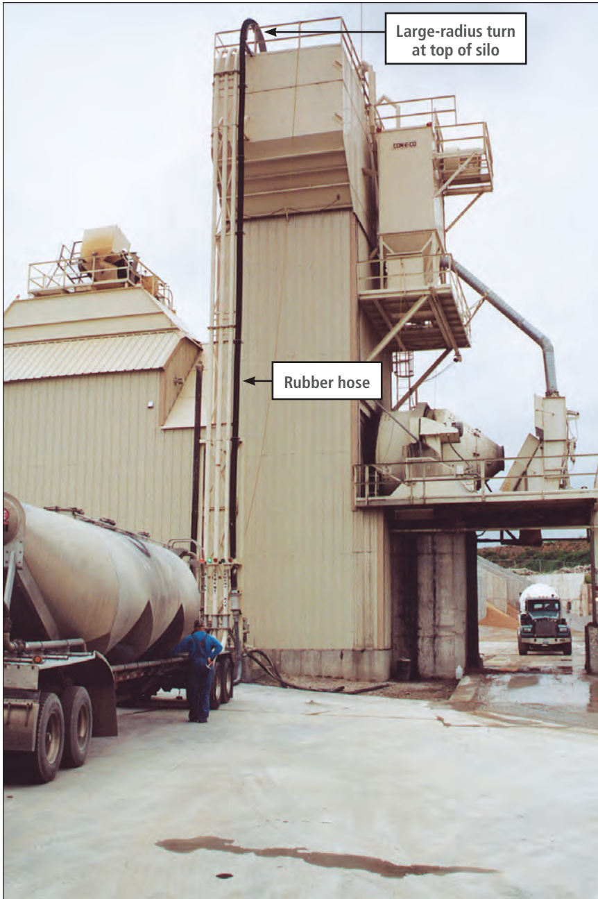
FIGURE 6.3. Unloading bulk densified silica fume into a silo. Note rubber hose and large-radius turn at top of the silo.
