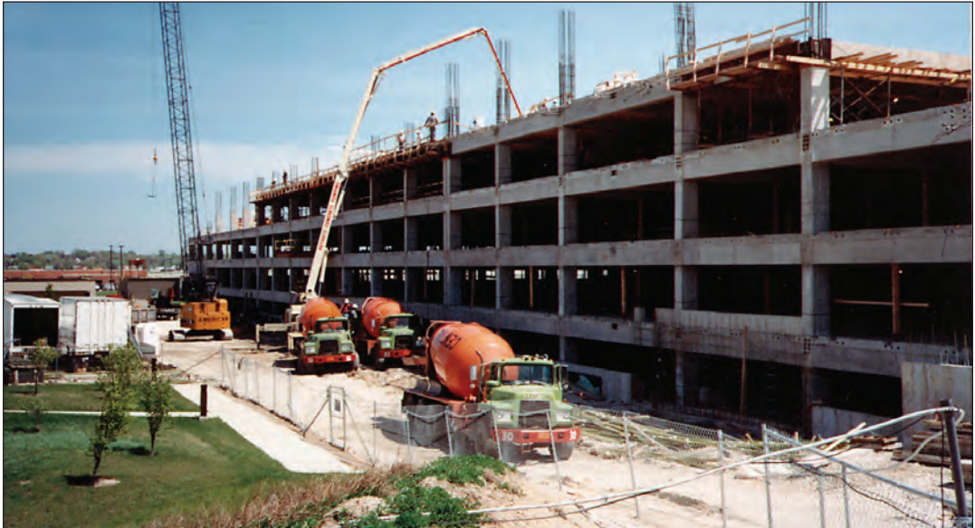
FIGURE A.2. Parking structure project. Mixture proportions for a concrete that could be used on this project are developed in Example 2.
