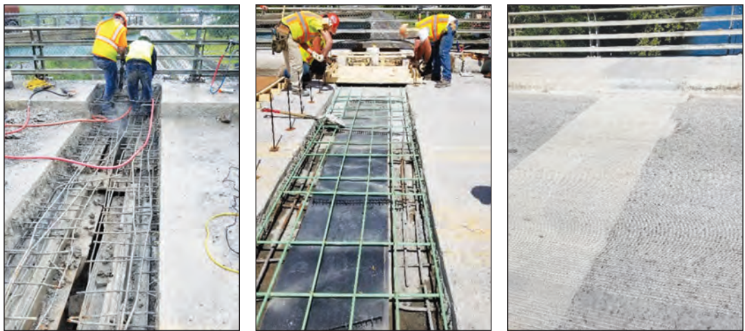
A B C FIGURE 3.21A, B, and C. Repair of a damaged bridge using a UHPC link slab. From left to right: A. Removal of deteriorated concrete; B. Link slab prepared for placement; and C. Completed repair. (FHWA 2022) (Photos copyright 2020 NYSDOT. Used with permission.)
