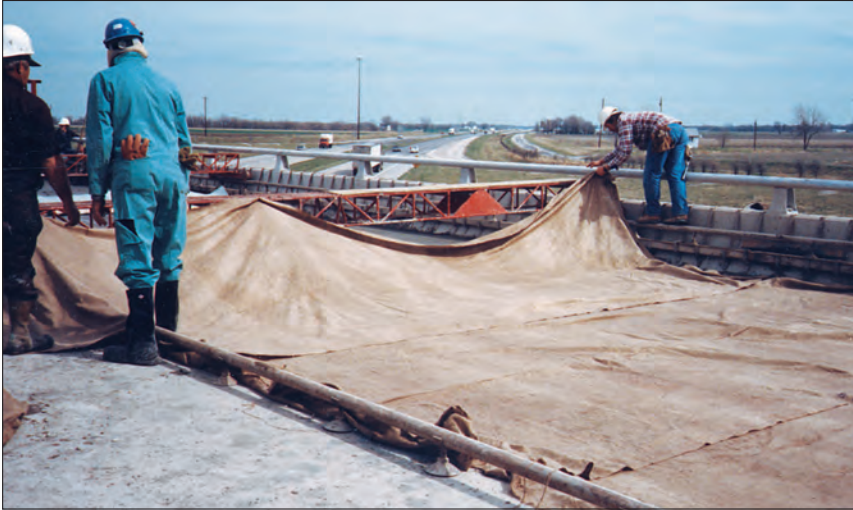
FIGURE 7.11B. Curing silica-fume concrete bridge deck. Applying wet burlap while the concrete is still too soft to walk on.
