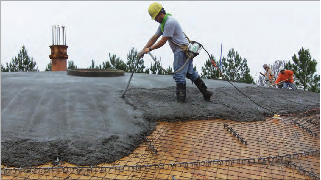
FIGURE 5.1. Silica-fume concrete being placed on the sloping dome of a waste-water treatment tank. Note the cohesive concrete holding the slope during vibration.
