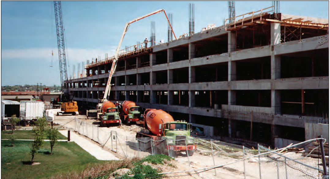
FIGURE 5.6. Parking structure project. Mixture proportions for a concrete that could be used on this project are developed in Example 2.
