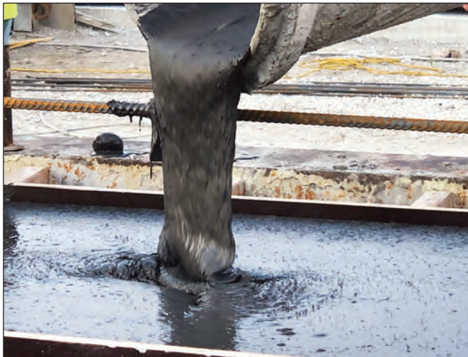
FIGURE 3.25B. The same beam being “topped-out.” Placed from a single point, UHPC’s high flow characteristics allow lateral void-less filling in a monolithic manner.
