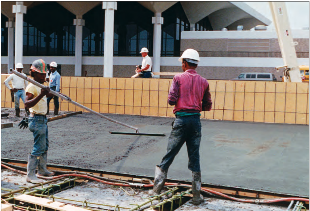
FIGURE 7.16. After screeding, the next finishing step is to bull float the concrete. Bull floating levels the surface and prepares the concrete to receive the texture desired.
