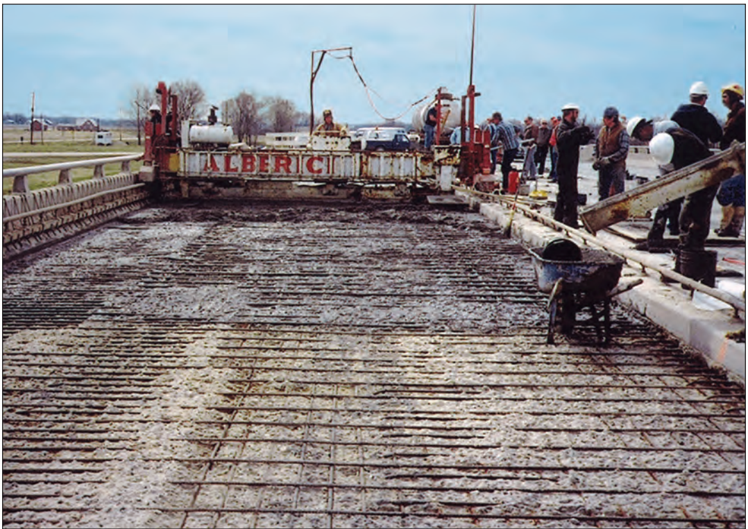
FIGURE 7.7. Concrete bridge deck prepared for a silica-fume concrete overlay. Deteriorated concrete has been removed and the reinforcing steel has been cleaned to prepare for the placement of the overlay.
