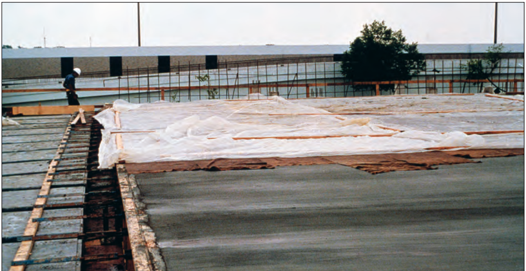
FIGURE 7.19. Burlap and plastic sheeting used for final curing. For most applications of silica-fume concrete, wet curing will provide better in-place concrete quality than the use of a curing compound alone.
