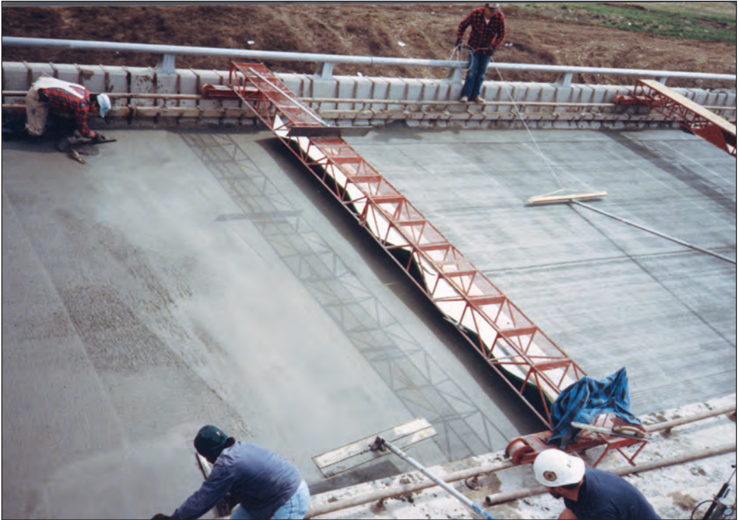
FIGURE 7.10A. Applying a broomed finish. After the finishing machine passes over the surface, some additional floating and finishing by hand may be required, particularly along the edges of the placement. Texturing using a broom can also be seen in this photo.
