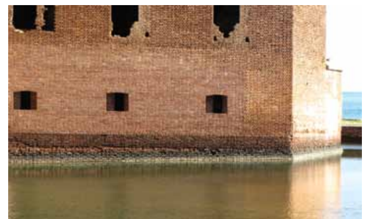
Figure 4: Settlements are as much as 24 inches per 200 feet. Here the water level in the moat makes settlement observation easy at Bastion 1.
