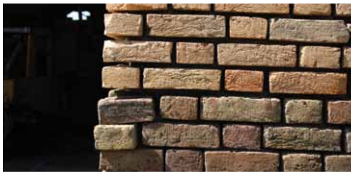
Figure 5: Mortar loss is severe in many areas.
