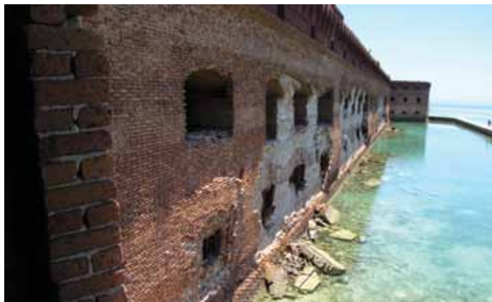
Figure 7: The damage to several fronts is severe but none as bad as that on Front 3.
