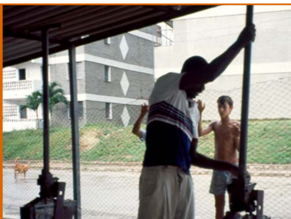
Photo 19. Manual Block-Making Machine Operated in La Güinera, with Five-Storey Standard Semi-Prefabricated Buildings in the Background
