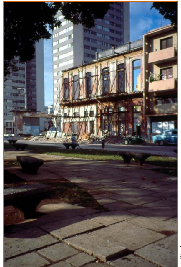
Photo 11: A Neoclassical Façade in Cayo Hueso, Shored Up after the Partial Collapse and then Demolition of the rest of the Building. Behind is a 20-Storey Prefab Apartment Building from the 1970's Urban Renewal Project
