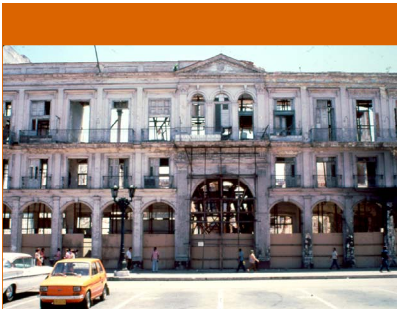
Photo 6: The Hotel Pasaje, a Century-Old Hotel Turned Ciudadela Housing 240 People Facing the Capitol Building in Downtown Havana, Collapsed in 1982
