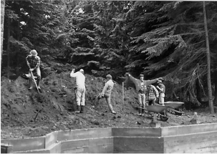
Backfilling the exterior of the foundation. Much work was done by hand rather than with machines.
