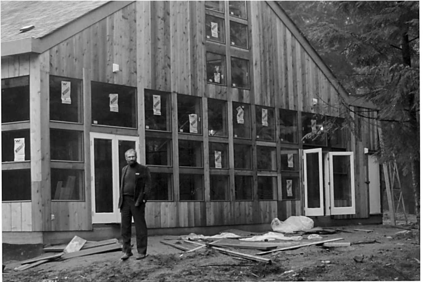
Allan Springman, chairman of the building committee, standing behind the unfinished building where work has come to an untimely stop due to a lack of funding for materials.
