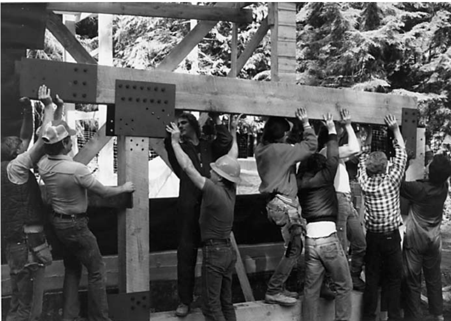
Trusses were made by hand on the ground. Drill holes (there were many) and plates had to match exactly. Crew is lining up the holes in a plate with the holes in a post.
