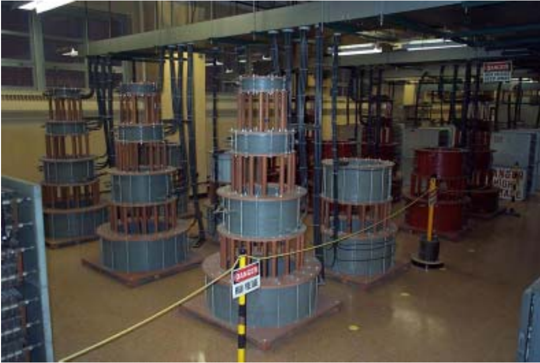
Figure 15. UL's Inductive Load Bank for Conducting Anti-islanding Tests.
