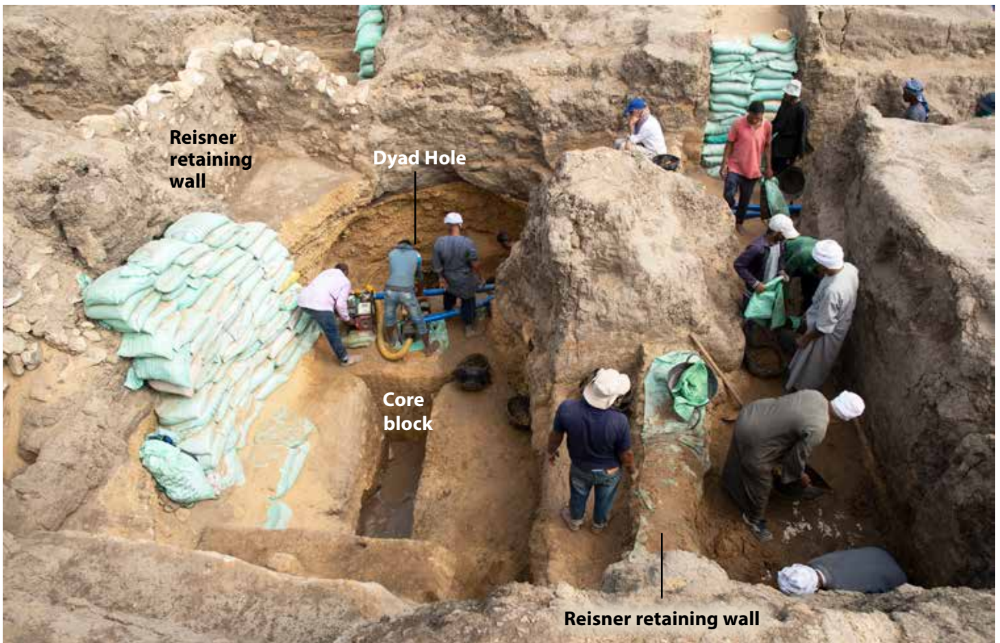
Above: Petrol generator being used to pump the water from the Dyad Hole. View to the east. Photo by Mark Lehner.
