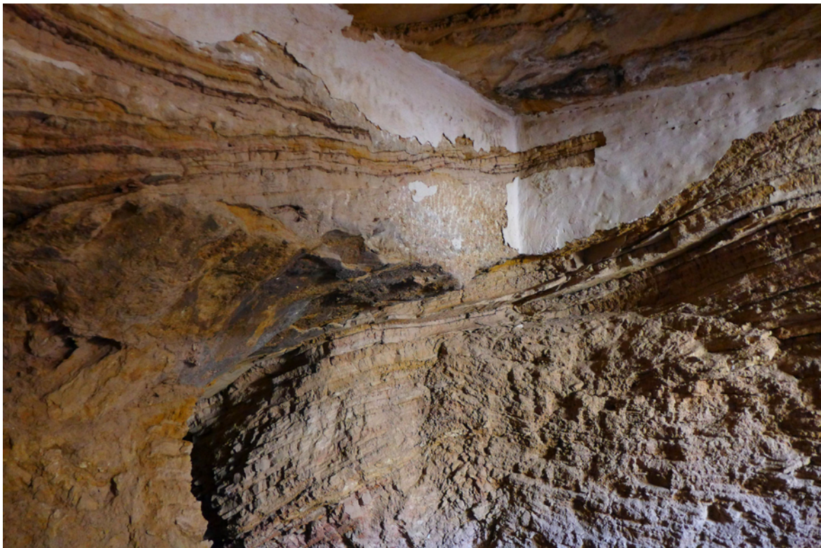
Figure 8. The ceiling in tomb 28, where the entrance corridor meets the descent to the rear chamber. The hard stone layer beneath the ceiling preserves areas of the original gypsum coating to all surfaces, which, for a time, would have concealed and helped to support the unstable rock surface below. Photo B. Kemp, 2015.
