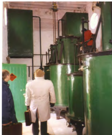
Fig. 10 Moyes equipment, Hurst Point Lighthouse
