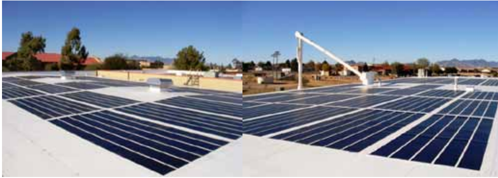
Figure 4. Two 30-kWp BIPV replacement flat roofs on the installation Library and a warehouse facility at Fort Huachuca, AZ.
