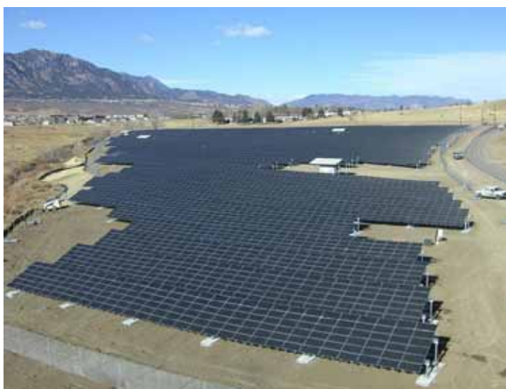
Figure 1. A 2-megawatt-peak (MWp) PV system at Fort Carson, CO.
