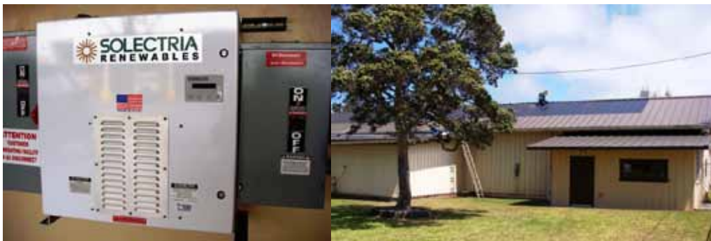
Figure 5. A 15-kWp pitched standing seam metal replacement roof on Bldg 84 at Kilauea Military Camp, HI. Also shown is the 15-kW DC-to-AC inverter at KMC Bldg 84.
