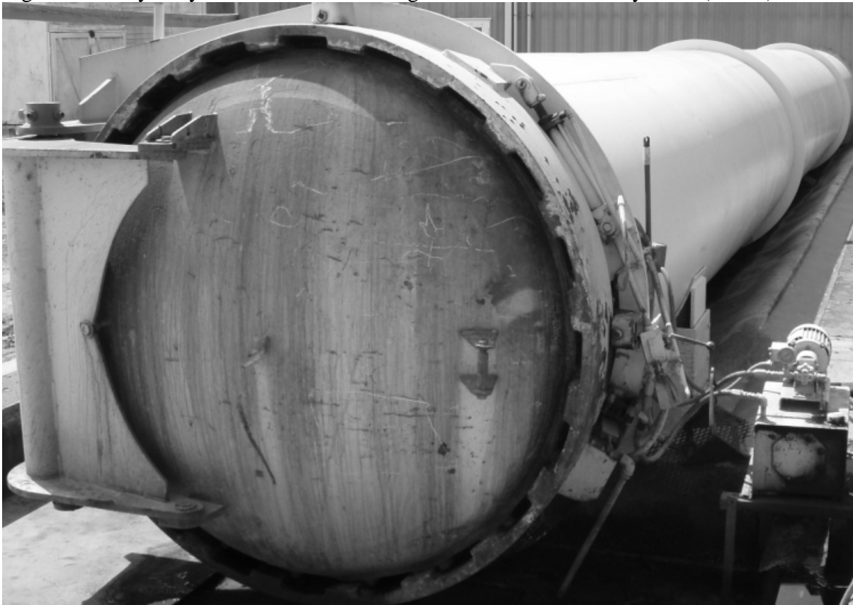
Figure 1. Heavy Duty Wood Preservative High Pressure Treatment Cylinder (Retort)
