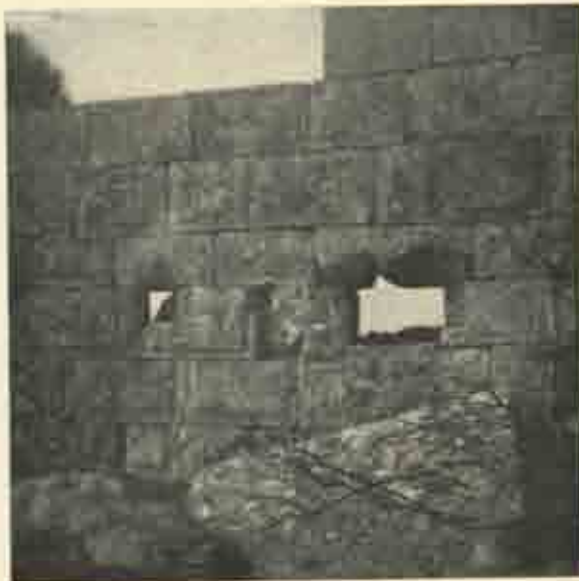
Wall of quadrated blocks with rough outer surfaces and drafted edges, at Dêhes
