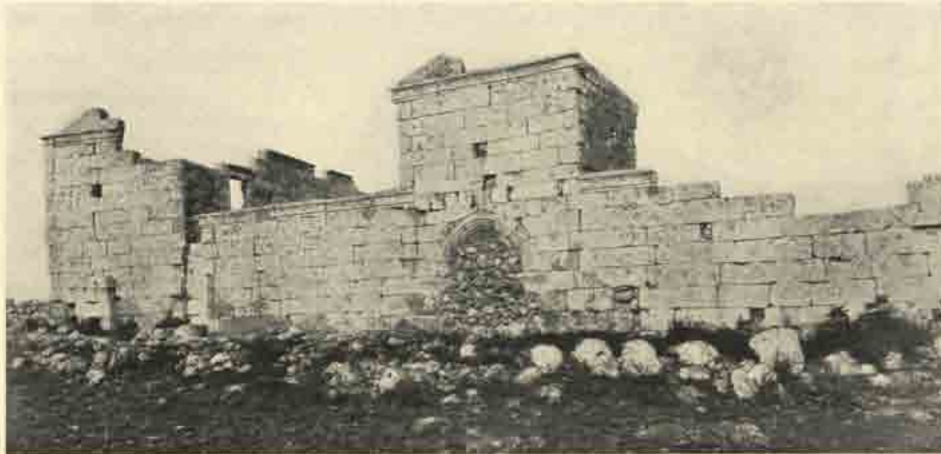
West wall of Villa I at Ruwēhā, showing arched entrance and tower.
