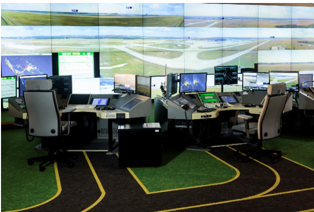
Figure Case Study 3: Inside the digital tower showing working positions Credit: HUNGAROCONTROL
