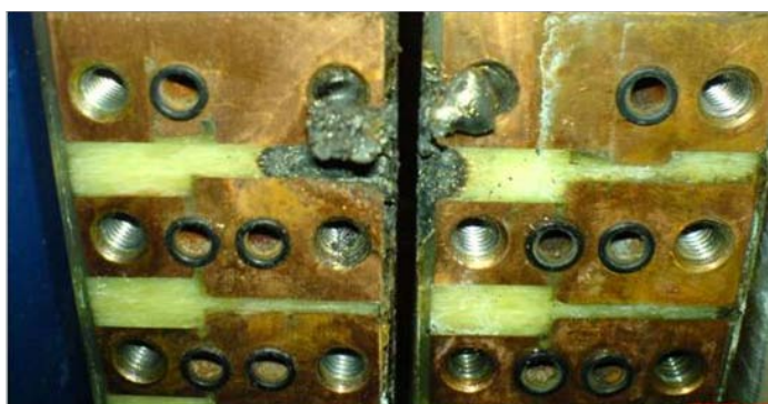
Fig. 10: A failure at a magnet connection post due to tracking triggered by humidity
