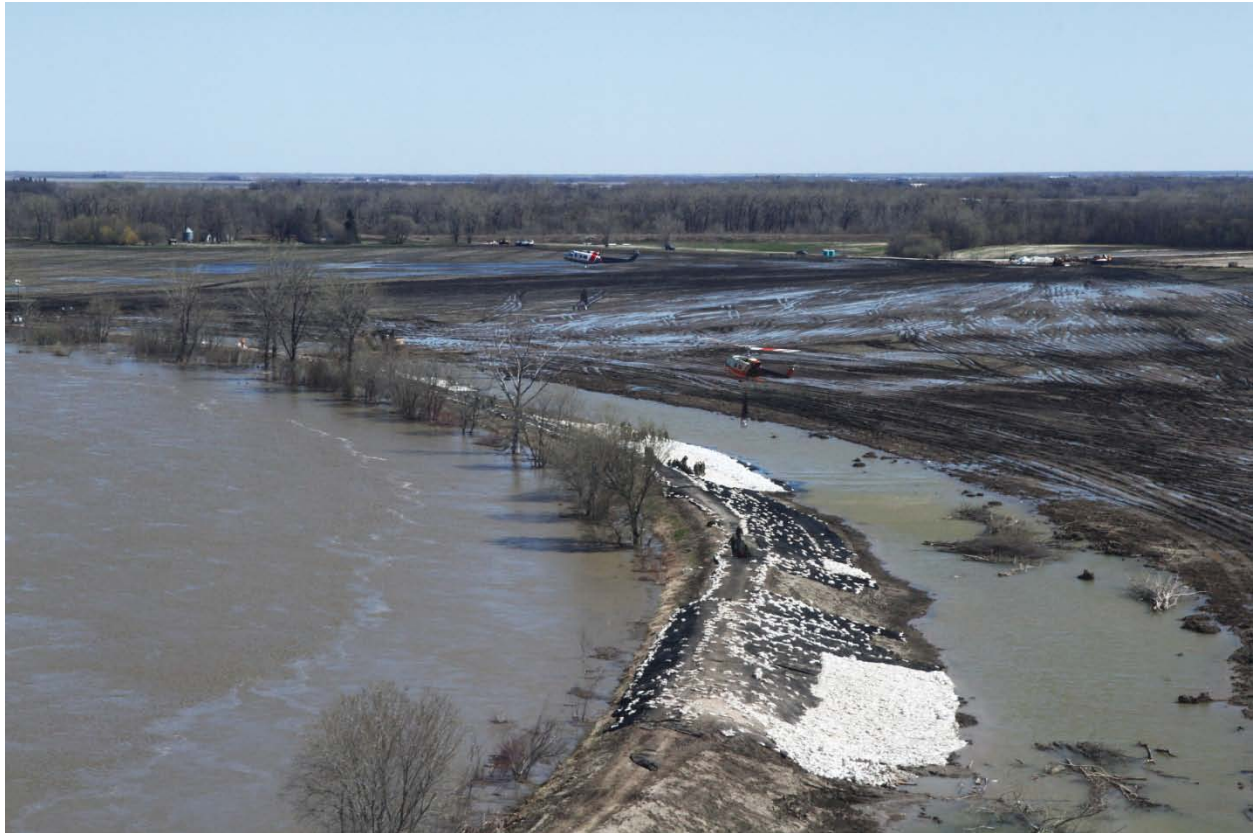
Figure 45: Photograph showing sandbags and filter cloth being used to shore up weak spots in the Assiniboine River dikes (photo from May 14, 2011).
