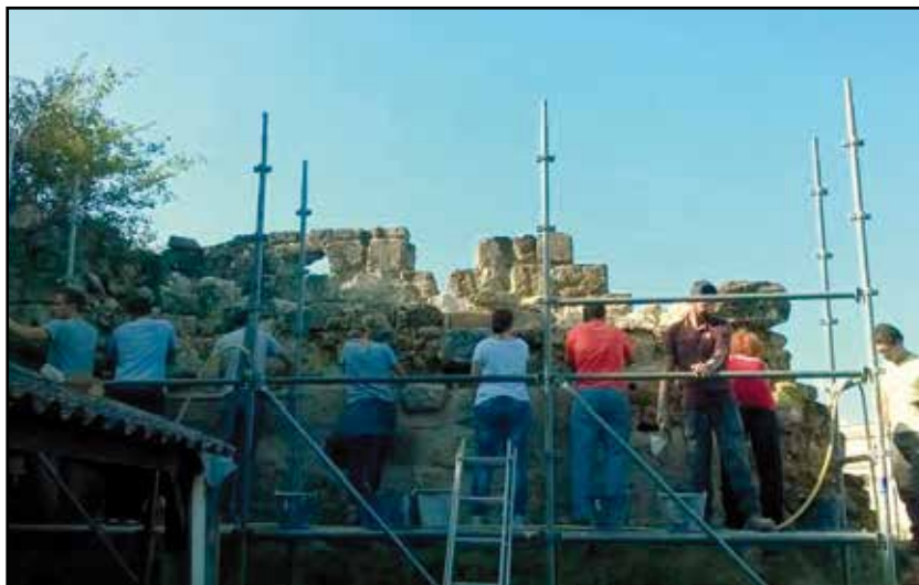
Maltese, French and Croatian volunteers working side by side on the part of the wall being restored
