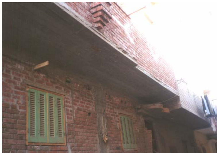
Figure 3-74 Building standards are not much lower than formal housing. The same building materials and finishes are used: a reinforced concrete skeleton with red brick walls.
