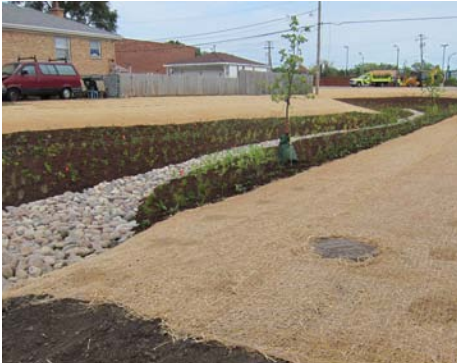
Bioinfiltration Basin in a Neighborhood Setting
