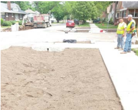
Engineered Soil in a Rain Garden
