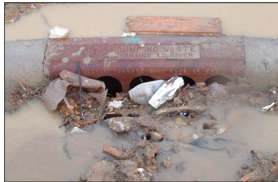
Figure 3-23. Accumulated sediment and debris at storm drain inlet marked “Dump No Waste; Drains to River.”
