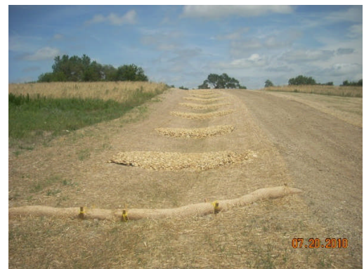
Figure 3-2. Soil Erosion and Sediment Control Practice: Rock and Straw Wattle Check Dams
