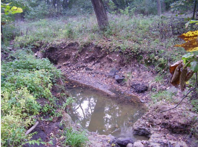
Figure 4-23. Channel downcutting and bank widening at Shaw Creek. Downcutting or vertical lowering of the stream channel is detrimental because it not only can increase bank heights and render them more unstable, but it can also contribute to undermining of the over-steepened bank, increasing erosion.
