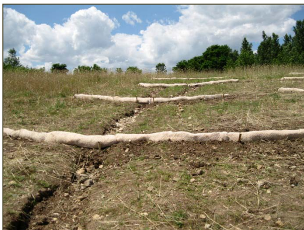
Figure 4-7. Although wattles were installed along a steep slope area, undercutting has continued to occur. It is recommended that rock checks be installed along existing gullies. In addition, a small berm could be constructed upstream of the gullies to store runoff and provide a potential mesic prairie / wetland restoration area. This would reduce runoff discharged to downstream areas and reduce potential gully erosion.
