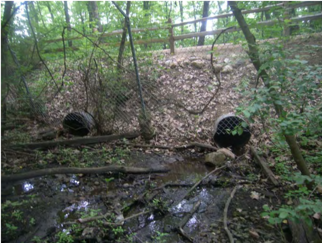
Figure 3-67: Example of a problem hydraulic structure
