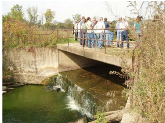
Lake County Forest Preserve will be removing the dam on Mill Creek that creates Rasmussen Lake and restoring the historic stream channel.
