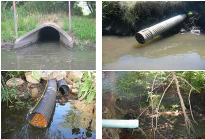
Figure 32. Examples of water discharges
