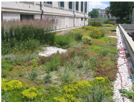
Figure 4.6 Example green roof.
